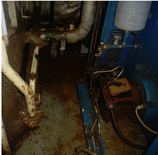
OLD DIESEL HOT WATER UNIT
